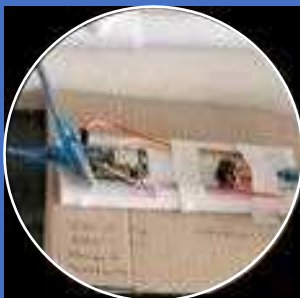
IOT Based Fire Alarm System
